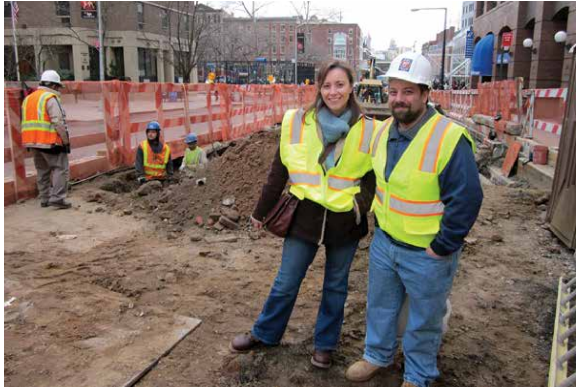
Opposite: Alyssa Loorya and Chris Ricciardi on-site at Fulton Street in lower Manhattan. This page, several artifacts excavated in the vicinity.
